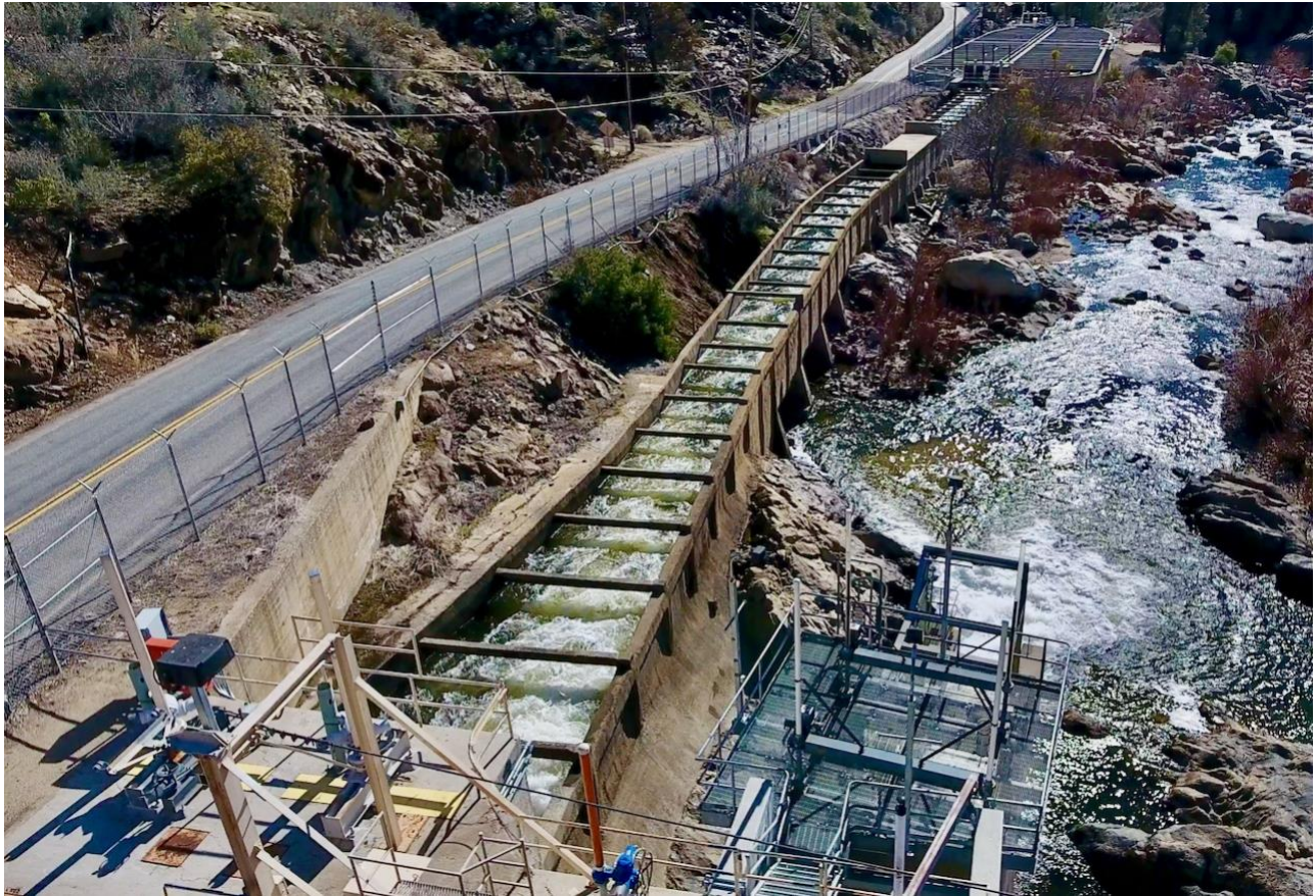
Figure 58: Edison removing about 550 of the available 600 cfs at Fairview Dam
